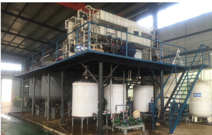
Actual MDS 1000 system for waste acid concentration
