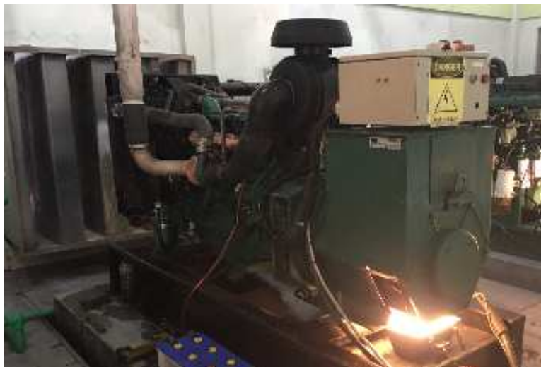
128 kw generator in the station
